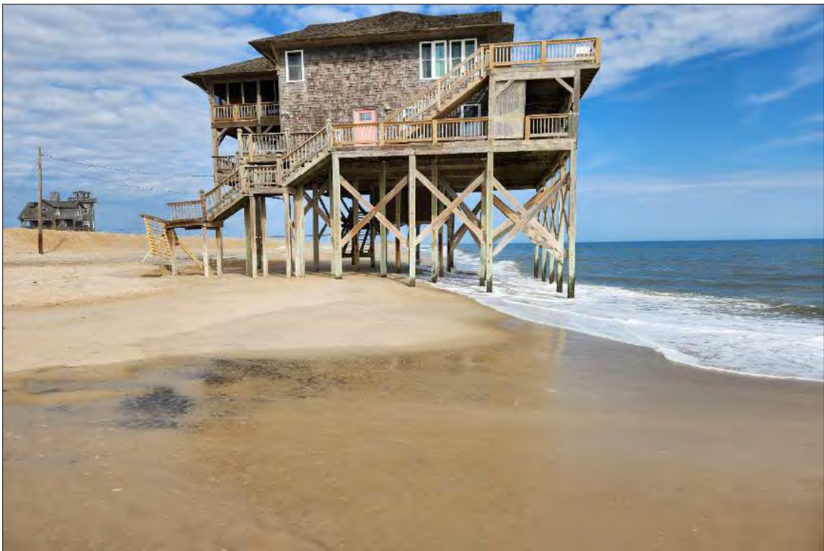
FIGURE 1.2b. Beach conditions along the Rodanthe reach offer little to no storm protection for many first-row homes, with several properties on the intertidal wet beach. The recent collapse of multiple such properties has compelled the County to investigate sand needs for a nourishment project at Rodanthe. The ground photo location is marked in the upper photo with a red circle.
