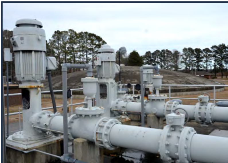
Water Treatment Plant
